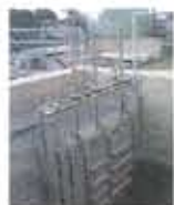
paratoie sluice valves
